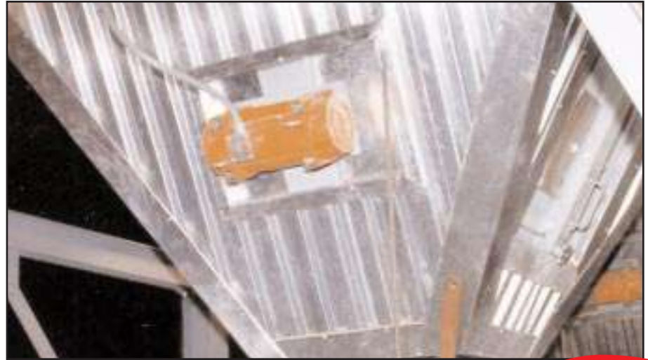
• SCR-500 on heat mount on hot ash bins
