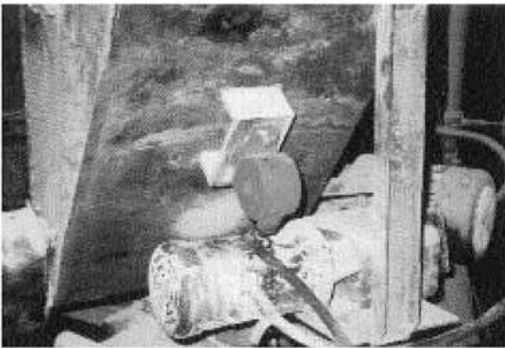
SILENT Turbine mounted to a fly ash chute to keep ash flowing.
