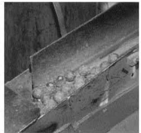
BVS-320 unjamming grinding balls on chute
