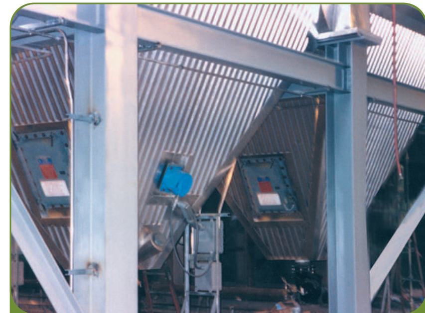
This Syntron® model V-85 Electromagnetic Vibrator is maintaining flow of dust particulates from the collecting hopper of an electrostatic precipitator.
